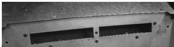
Fig 4 - Flue Restrictor Baffle Not Fitted
