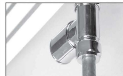
8. Run the central heating to the radiator
